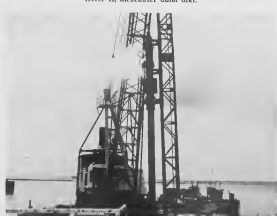
THE STEAM driven pile driver goes to work on the first pile. The ram is lifted by steam but drops free. Its 12,500-pound weight generates 40,650 pounds of energy in a thirty-nine-inch fall.
